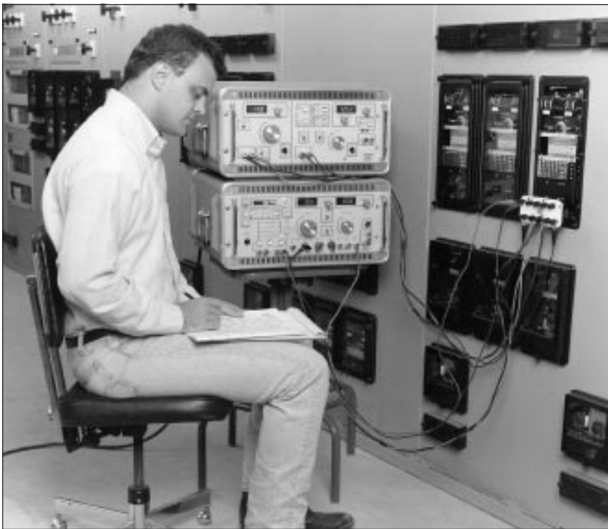
Model SR-90, with Units 1 and 2 stacked, tests a current differential relay in a panel.
