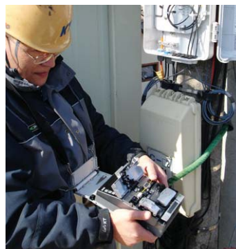
On a Telephone pole
