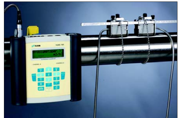
Measurement with transducers mounted by mounting frames and flow transmitter fixed to the pipe by the QuickFix pipe mounting fixture
