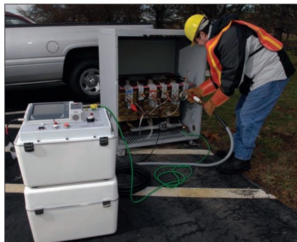
DELTA3000 shown testing a pad mount transformer
