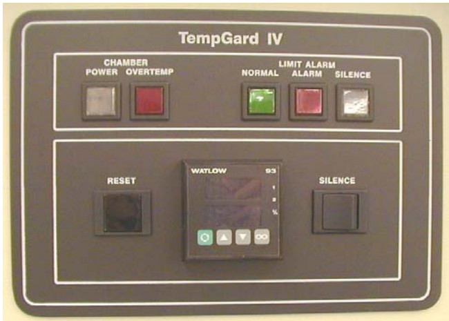
TempGard IV Panel
