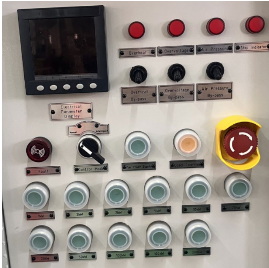
Control panel for reference
