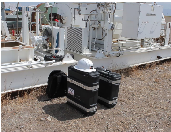
Staging the iTIG IV and Power Pack before field testing pump motors at Power Zone Equipment, Inc.
