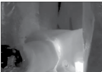
Leak in a 4-way valve dryer skid
